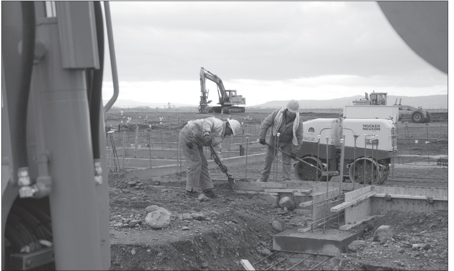
Crews prepare the necessary forms for the concrete foundations of the future Kootenai Technical Education Center (KTEC) under construction at Lancaster and Meyer Roads.
