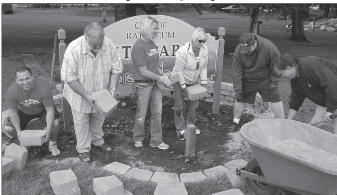
As part of their annual United Way Day of Caring program, four top executives of the Coeur d'Alene Fred Meyer store pitched in last Thursday to build an attractive rock planter around the entry sign at City Park. The four executives plus Mayor Vic Holmes (second from left) and Park and Recreation Director Lance Bridges (right) are Store Director Bob Hobart; Human Resources director Tanna Kluss; Operations Manager Eve Cluster, and Loss Prevention officer Brandon Nason. Fred Meyer, reported Hobart, allows "selected employees the opportunity of going into our neighborhoods and volunteering their time to help in constructive ways. Today we selected Rathdrum, largely because good things are happening in that city and we wanted to be a part of it."
