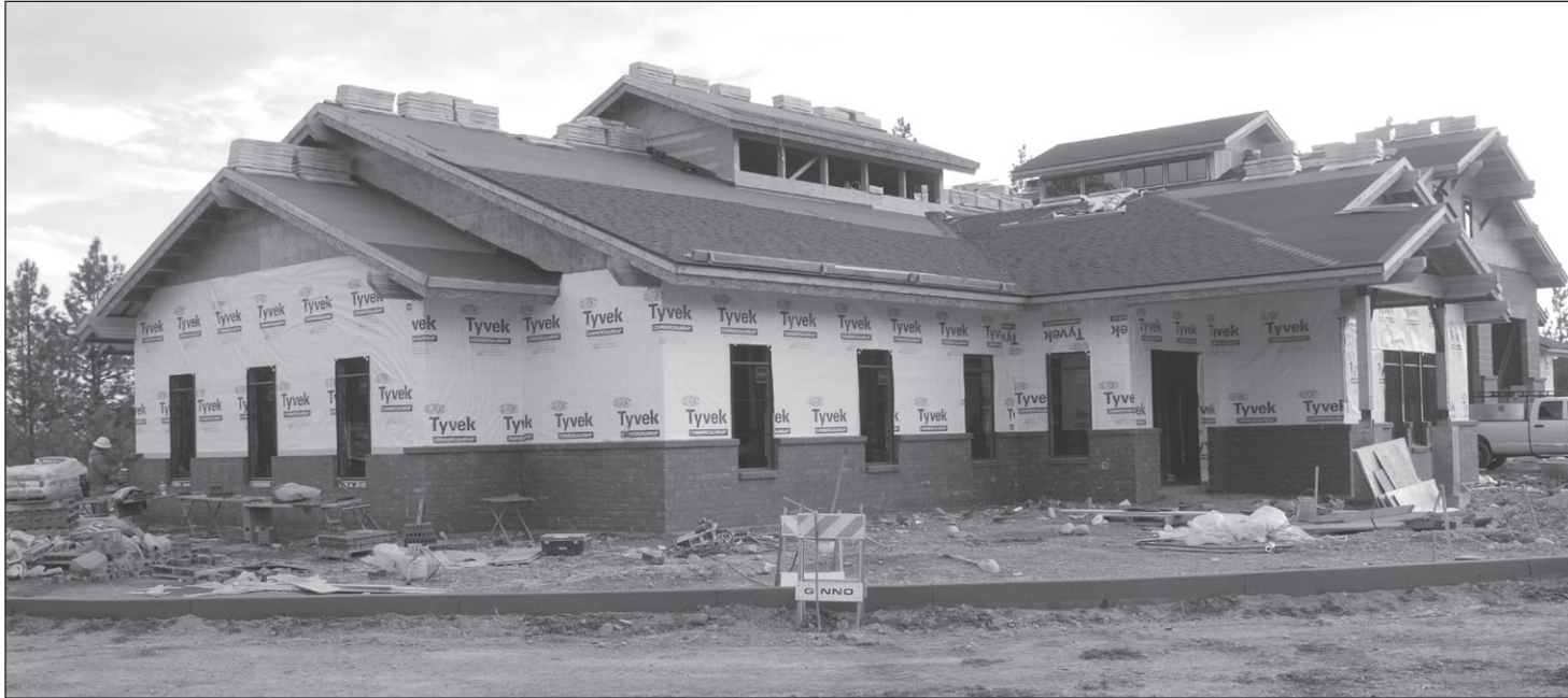
Construction continues on the new, $2 million Northern Lakes Fire Station on Highway 53. Barring inclement weather, the building is expected to be finished by December.
